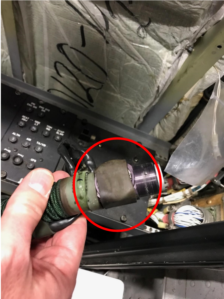
Anti-Suffocation Valve Covered
